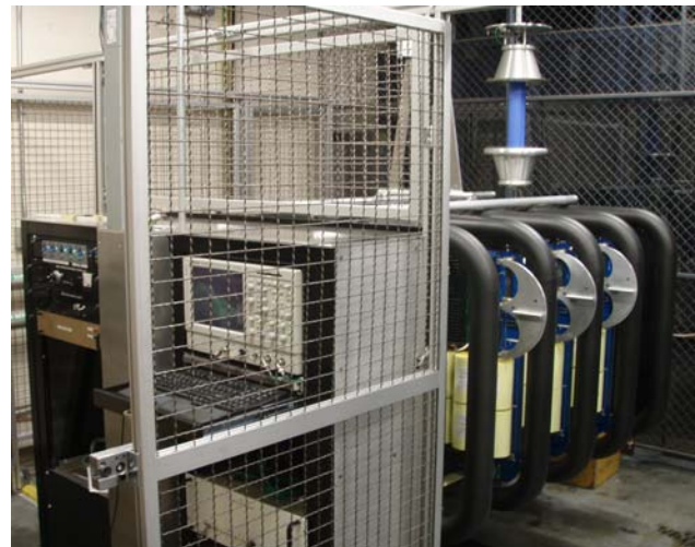
Figure 1. The ILC Marx Modulator in Testing Area.
