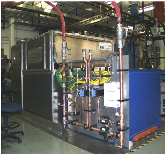
Figure 2. Converter Modulator Assembly
